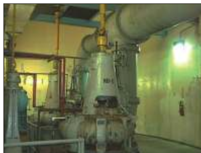
JEA Grove Park Pump Station
