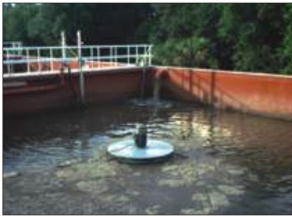
Labelle wastewater treatment plant reactor
