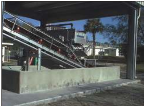
Wastewater treatment plant belt press
